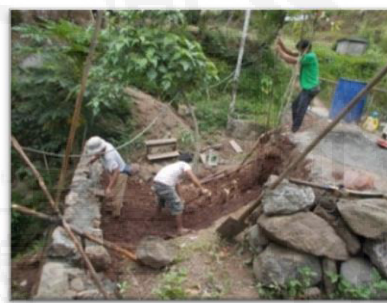
Figure 23 The indigenous skills of stonewalling is a paid labor used in this government project.
