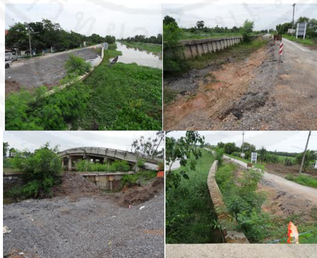
Figure 4 Concrete fence for canal landslide protection in Thailand
